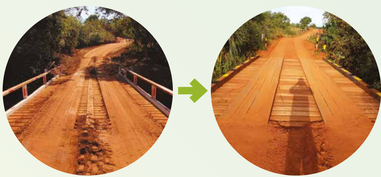
Bridge in Barraca farm and bridge that access Barra da Boa Vista farm.
